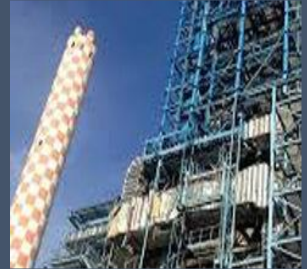
HFO Fired Power Plant, Cyprus
